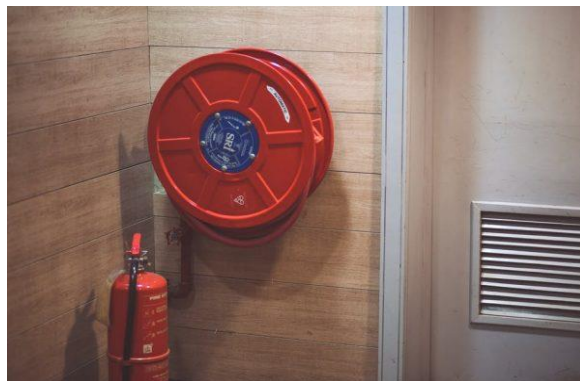
Figure 6. Fire extinguishers and hydrants
